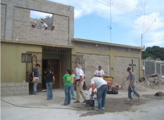
Teams worked to put three rooms atop Promesa de Vida 's building.
